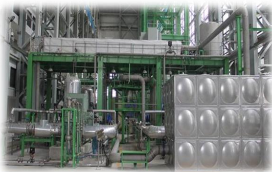
Integral Scale Hydraulic Test Facility, ISHY
